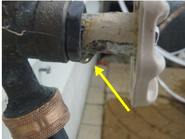
rear hose bib was leaking. Repaired by inspector.
