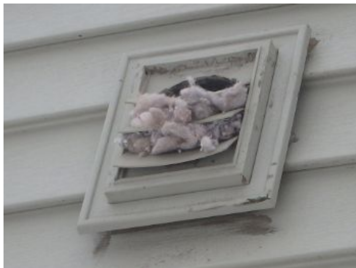
Dryer duct was plugged. Cleaned by inspector as a courtesy.
