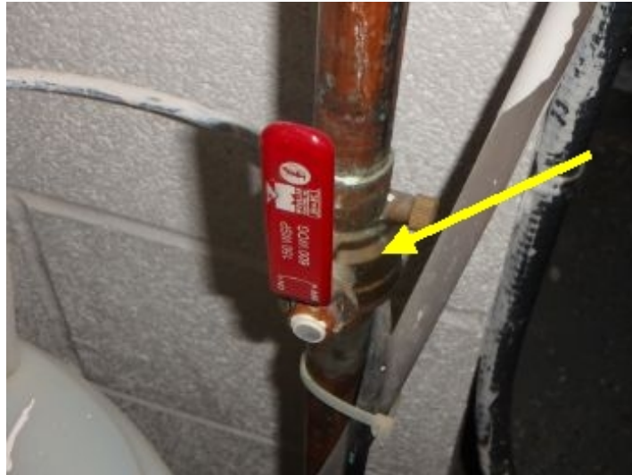
Main water shutoff.
