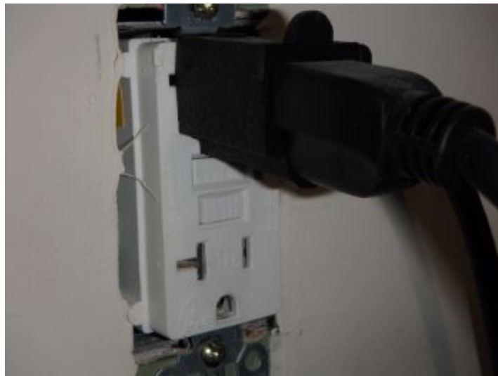
Missing cover in basement.
